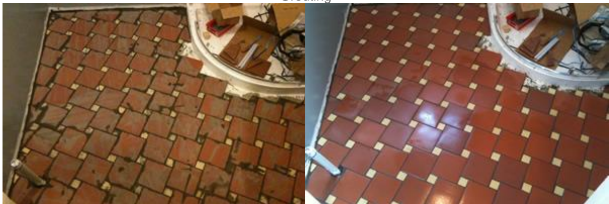
Letting the grout dry and cleaning the grout with a sponge and clean water (and nothing else)
